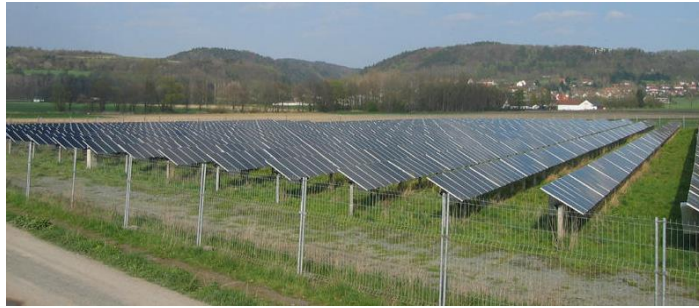
Figure 2. Module tables oriented towards the south.
