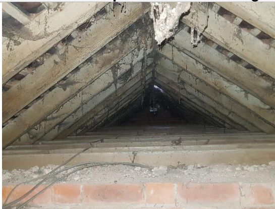
Plate IX. Roof void looking northward. Gaps showing along the ridge, toward the gable wall.
