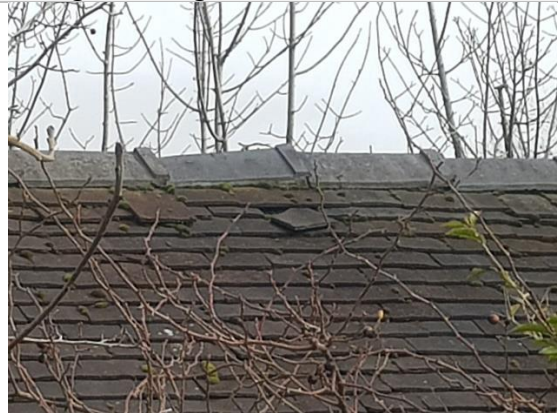
Plate IV. Multiple gaps where mortar has failed under ridge tile and cracked and missing common tiles.
