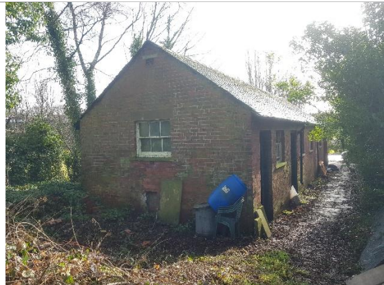
Plate II. Northern gable with missing bricks at the base and missing mortar along the verge.
