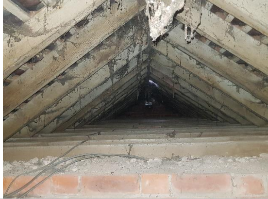
Plate VIII. Roof void looking northward. Gaps showing along the ridge, toward the gable wall.
