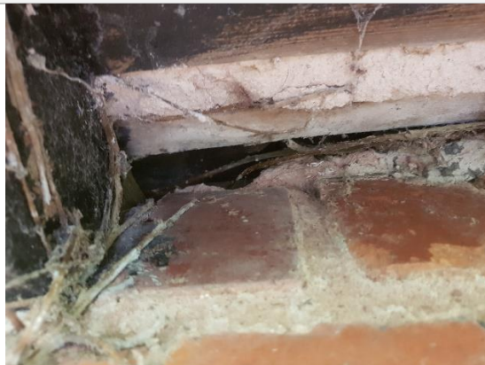
Plate V. Gaps at eaves with access into roof void.
