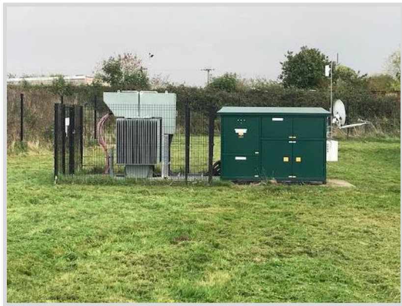
Figure 4: Typical LV Switchgear with Transformer
