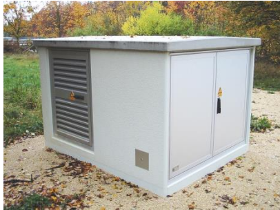
Figure 5. Example of a 20 kV / 400 kV transformer station.
