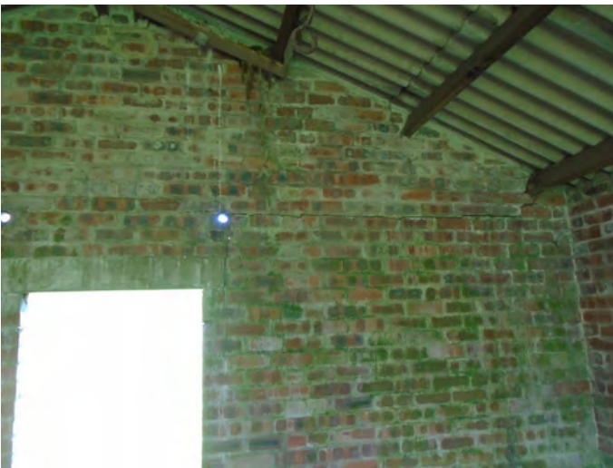
Building C. Cracks from corroding embedded metal (tubes).
