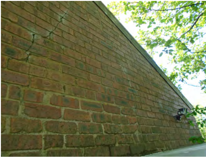
Building B. Cracks to gable.
