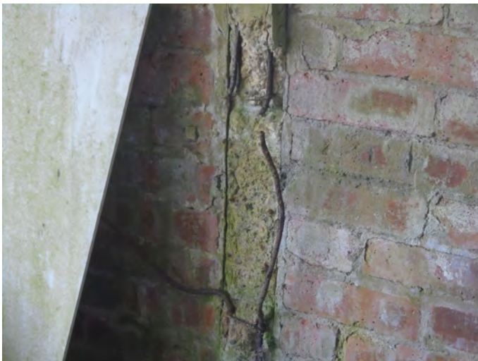
Building D. Internal cracked concrete and exposed reinforcement.
