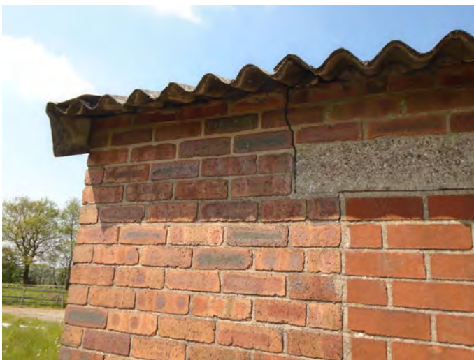
Building B. Minor cracks to brickwork – typical of all buildings.
