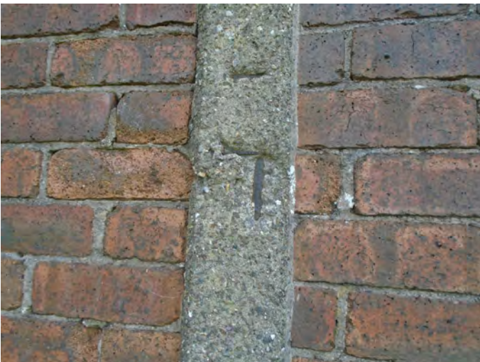
Building D. External exposed reinforcement to columns.
