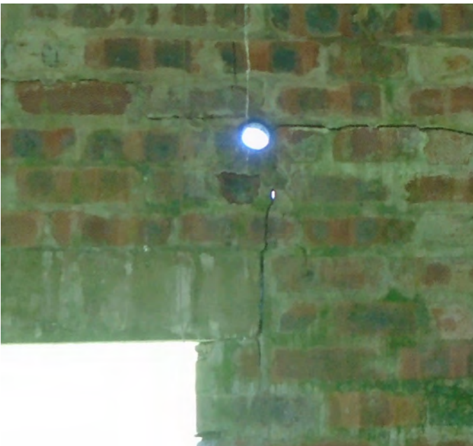
Building C. Close-up of cracks from embedded metal.
