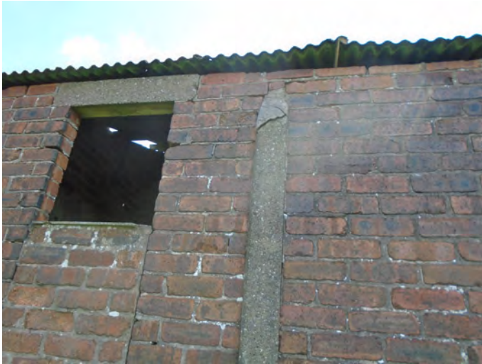
Building D. External cracks to columns.
