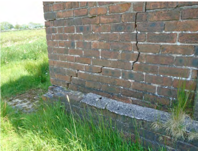
Building D. Significant cracks – North end of the West elevation.
