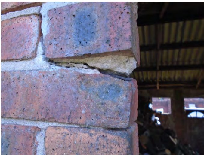
Building A. Corroding embedded metal causing cracks to brickwork.
