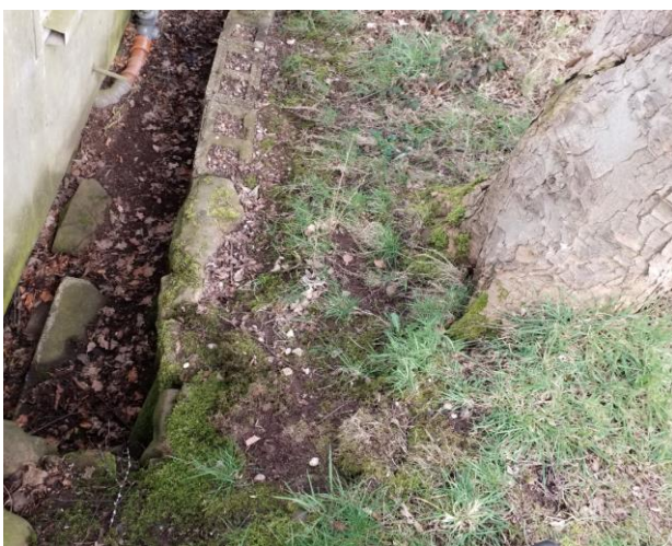
Fig 6: T2 making the retaining wall bow.
