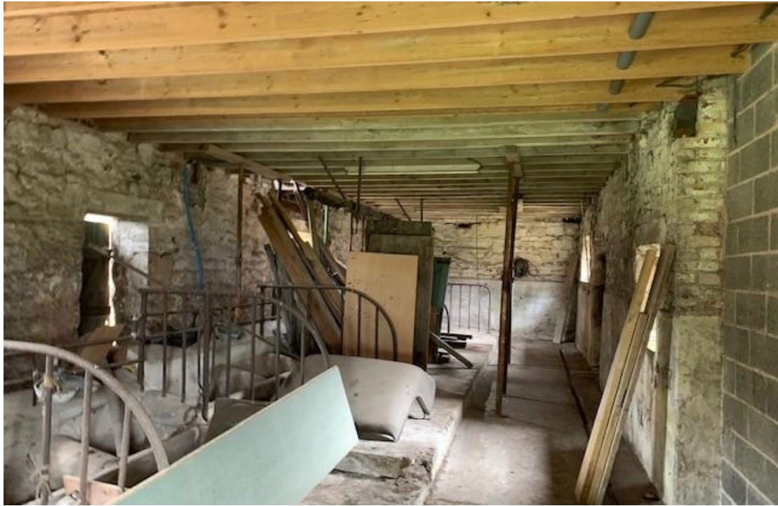
Timber first floor with south east section – note acro props supporting defective floor sections.
