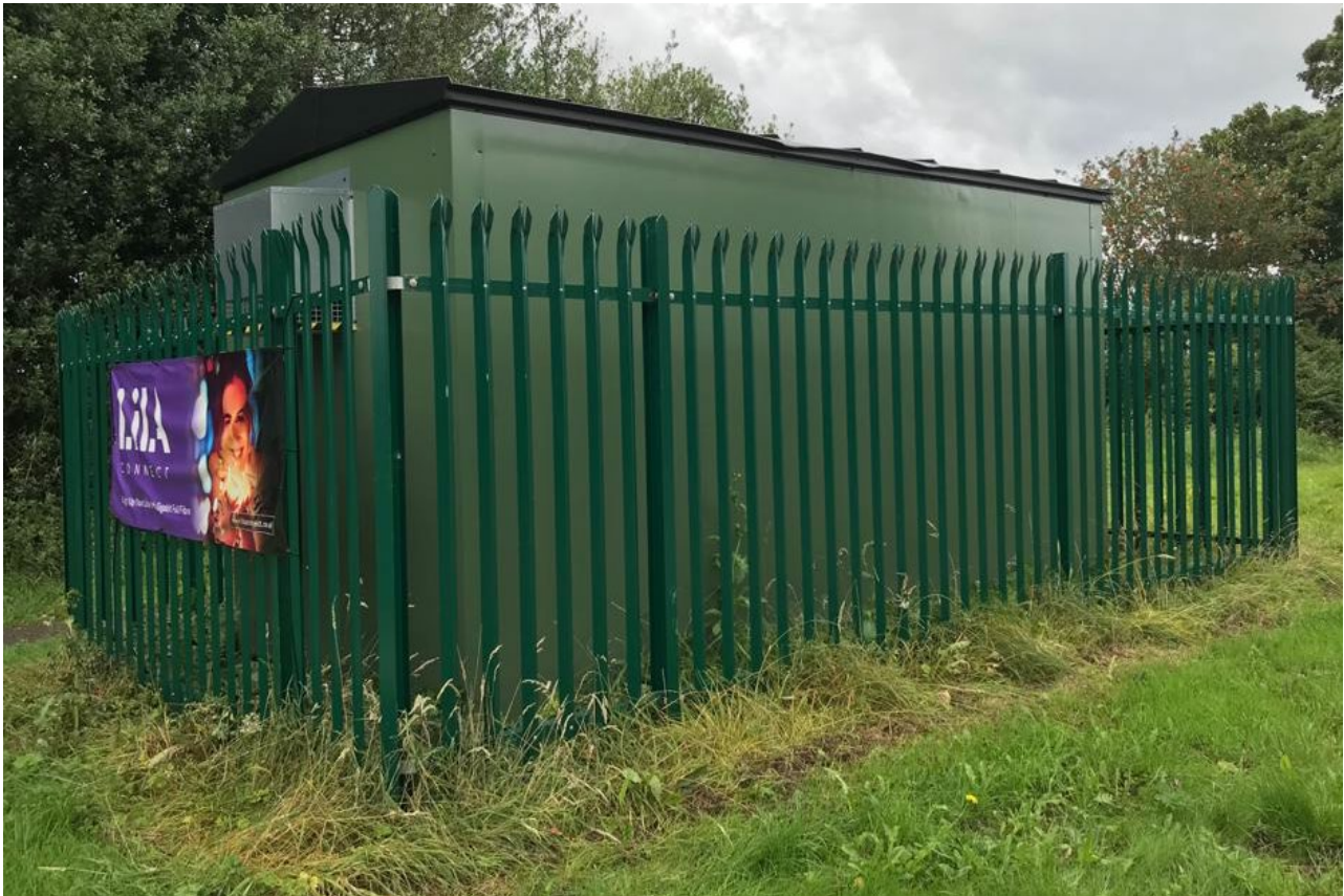
Photograph 1: Telecoms Shelter and Security Fencing in situ
