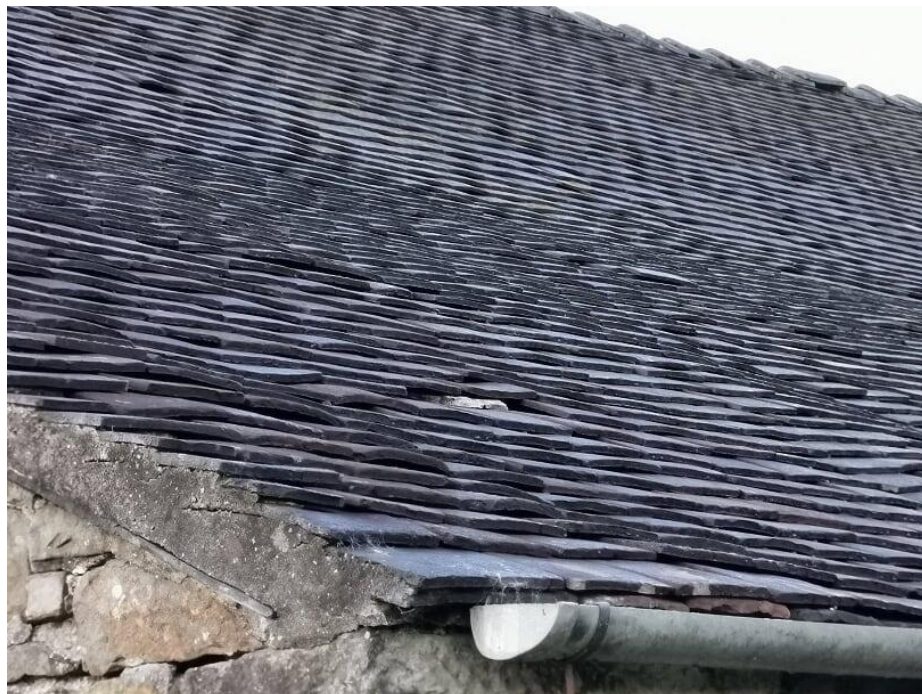
Plate 2: An image showing the missing and lifted tiles on the roof of the barn.
