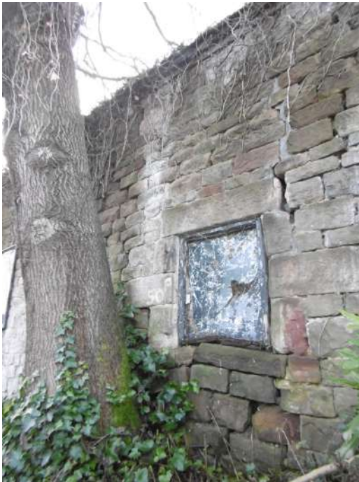
Eastern canal side wall with tree causing severe cracking to wall and foundations
