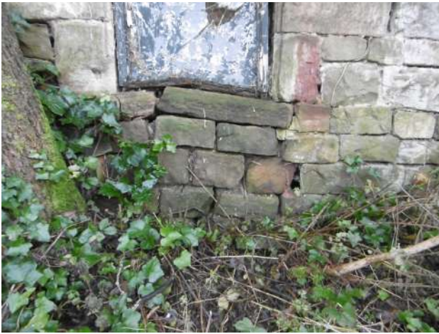
Distorted and cracked wall under window
