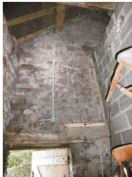
Internal wall over basement door with cracking over right hand side of timber lintel
