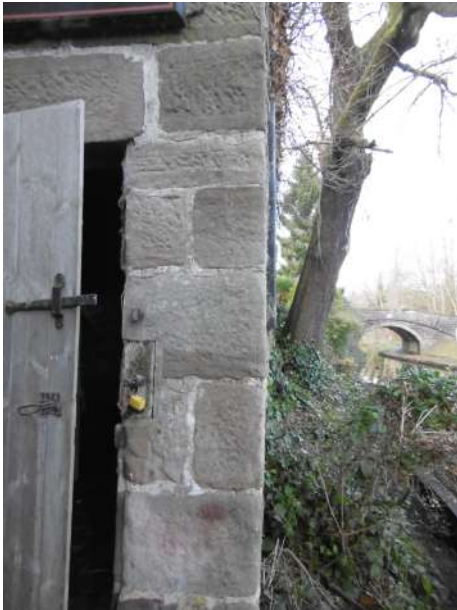
Basement door with poorly supported lintel and leaning tree alongside canal
