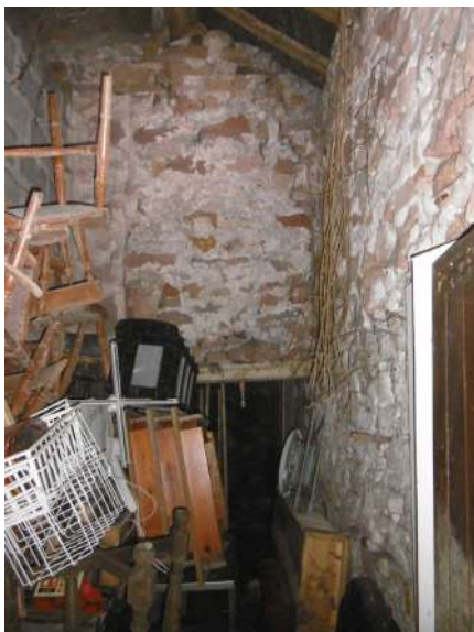
Internal passage with opening to rear basement with defective timber lintel supporting stone wall
