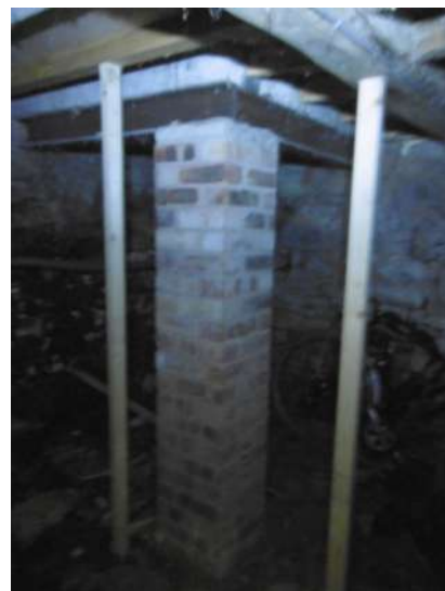
Brick pier in rear basement and timber props supporting cafe floor
