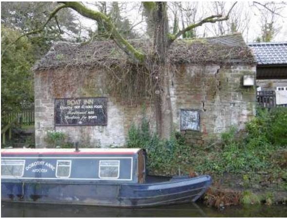
Eastern canal side wall with tree causing severe cracking to wall and foundations
