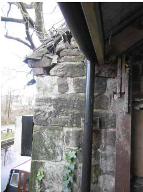
North elevation gable showing loose stonework at eaves
