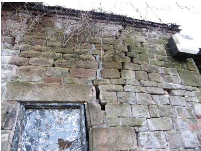
Severe cracking to wall above window having been repointed and since re-cracked
