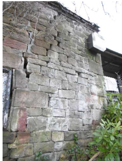
Severe cracking to wall above window having been repointed and since re-cracked
