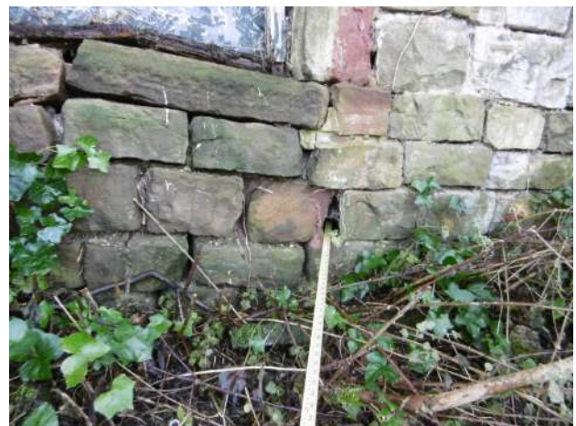
Distorted and cracked wall under window
