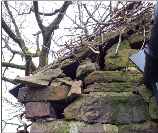
Plate 6: Photograph showing the large cracks within the brickwork on the north-east gable end.
