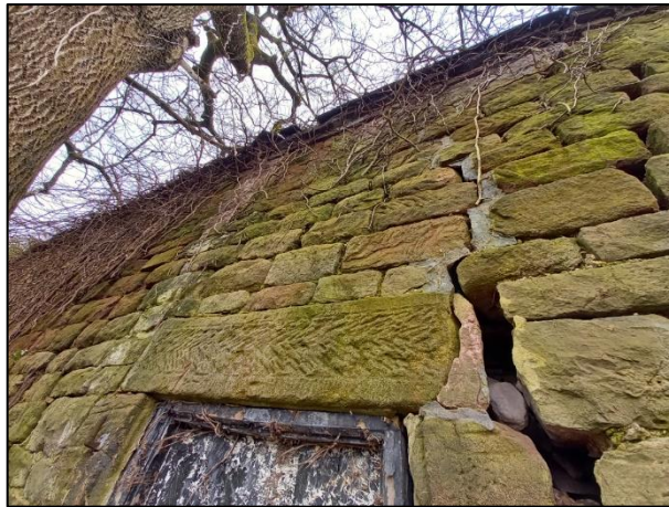
Plate 7: Photograph showing the large crack on the eastern elevation of the building.
