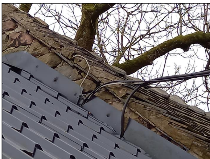
Plate 5: Photograph showing the gaps between the tiles and the wall top on the southern gable end.
