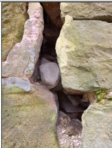
Plate 9: Photograph showing the depth of one of the cracks present on the eastern elevation.
