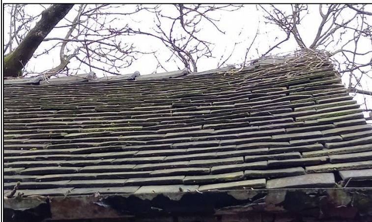
Plate 4: Photograph showing the lifted and warped slope and ridge tiles on the store building, Boat Inn.
