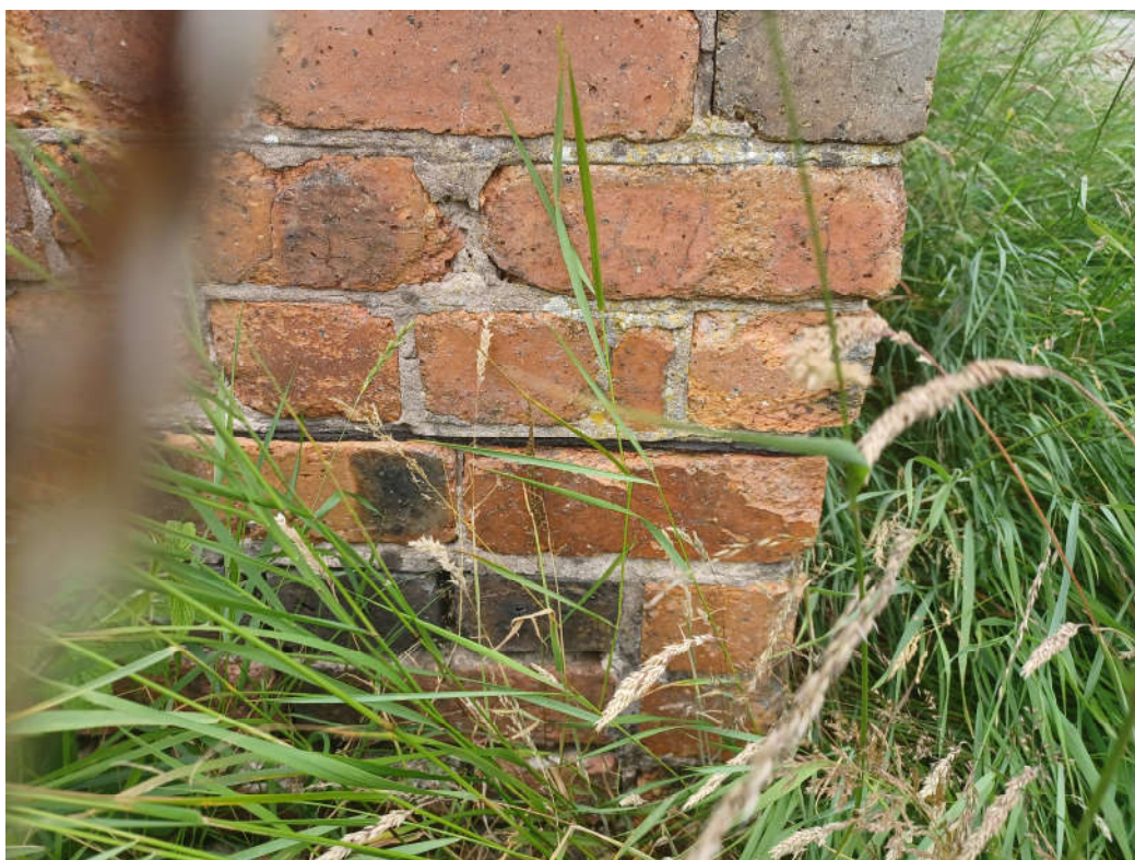
Photo 11 Brickwork to right hand side of rear wall oversailing DPC
