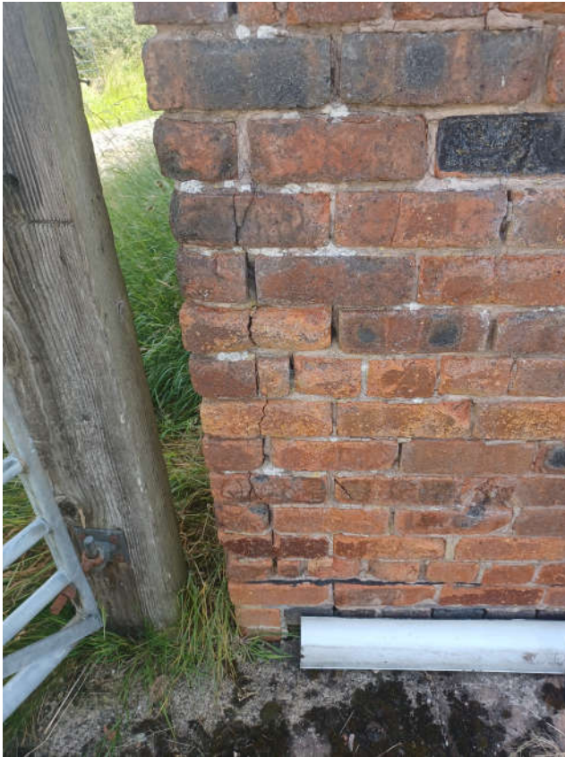
Photo 3 Front elevation crack to brickwork
