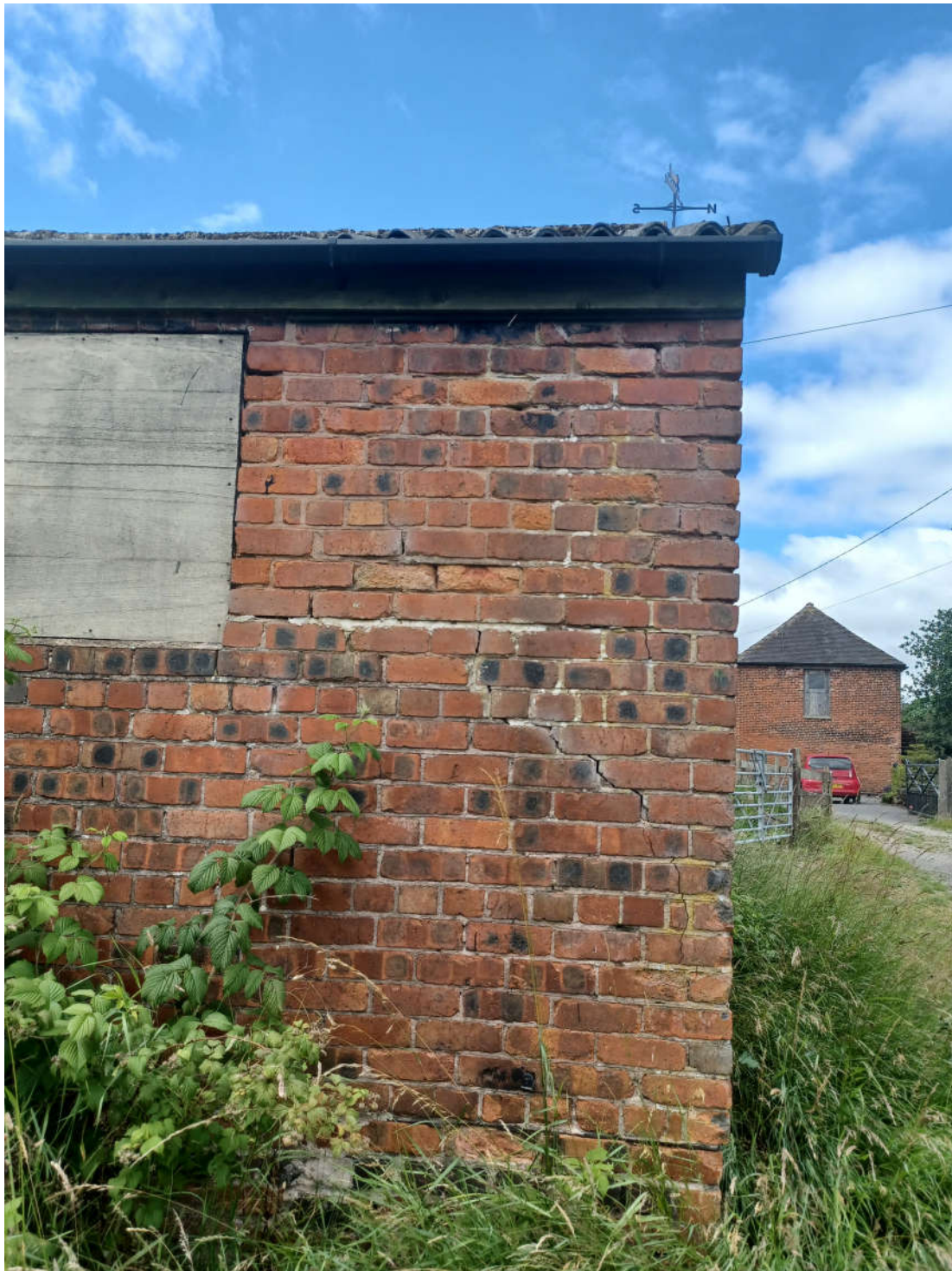
Photo 9 crack to rear wall
