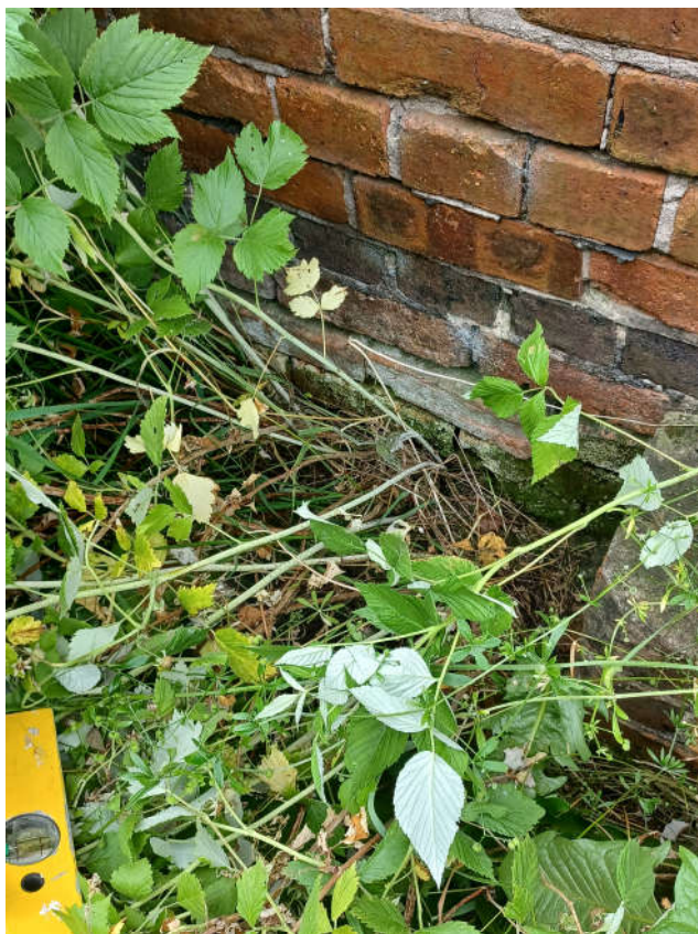
Photo 8 defective brickwork below DOC to rear wall
