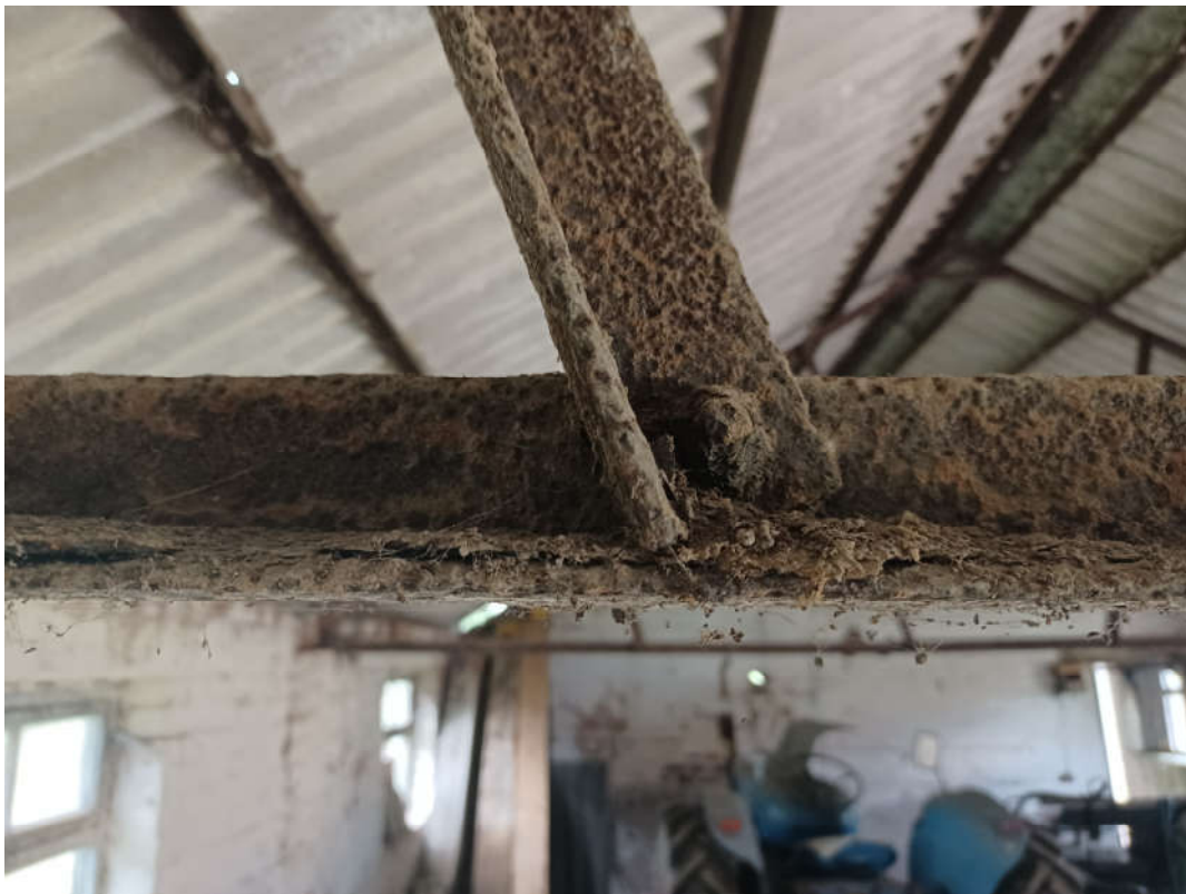
Photo 15 corroded hot rolled steel trusses and connections
