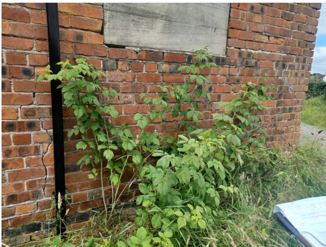
Photo 10 Crack to rear wall
