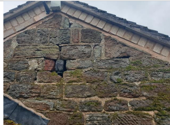
Plate VI. Missing mortar around the blocked ventilation hole at southwest gable of shippen.
