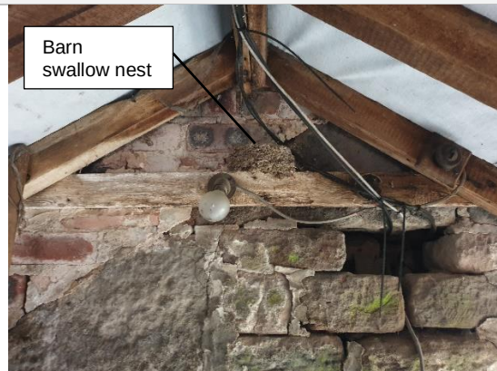
Plate X. South western gable wall of shippen within the pigsty, showing gaps in stonework.
