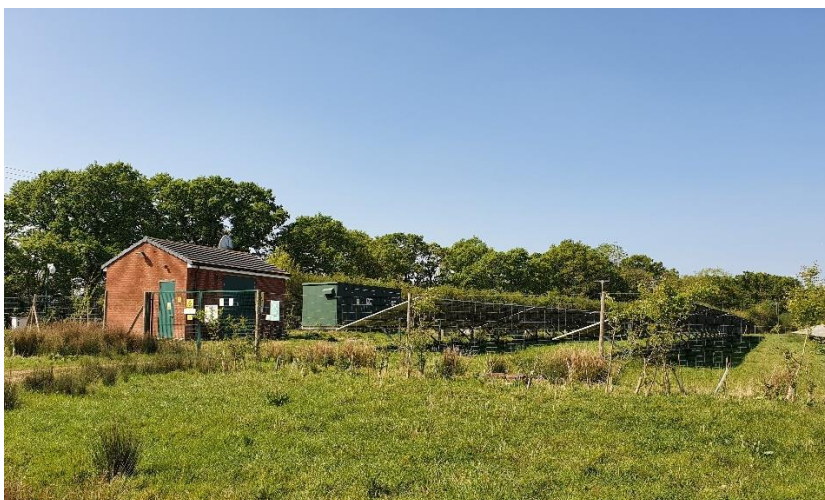
Example of a brick substation building and inverter/transformer cabin
