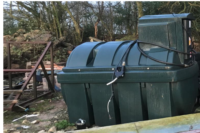
Above Ground Fuel Storage Tank (AST)
