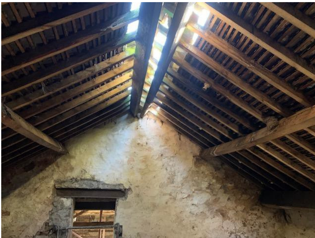
Internal view of brick work barn showing missing tiles at the ridge
