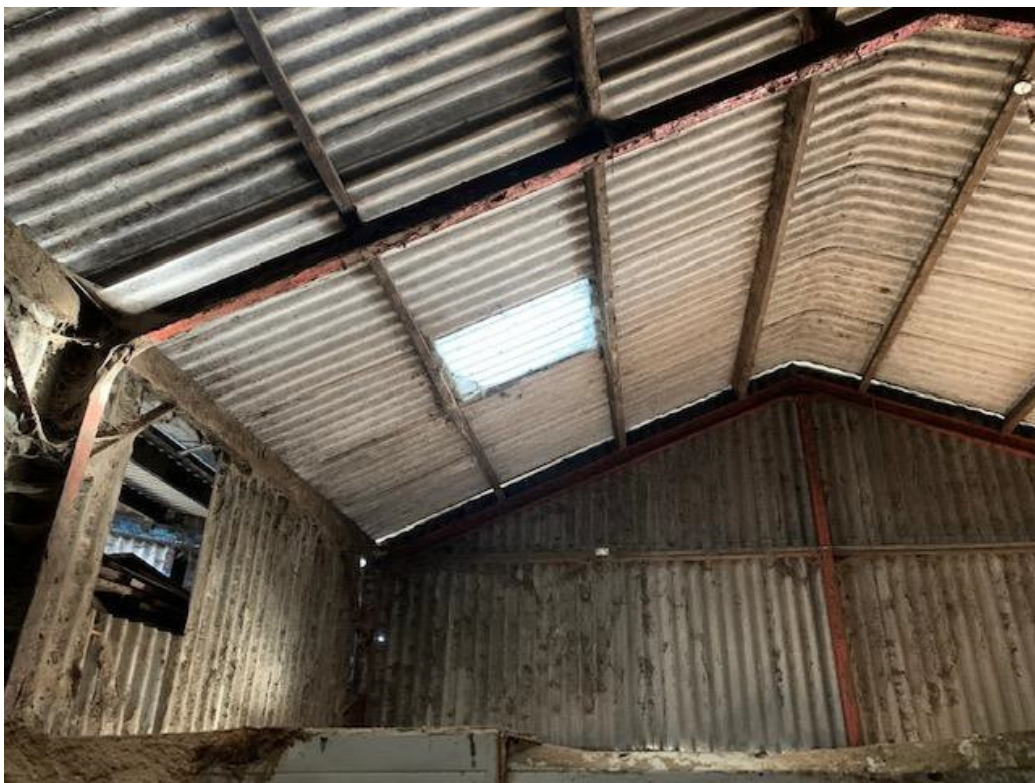
General internal view of smaller portal framed building with surface corrosion to steel elements.
