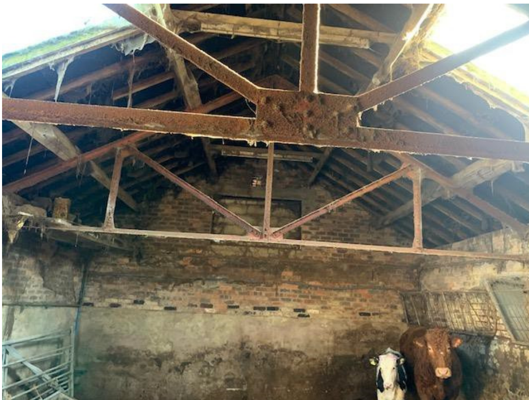
Masonry barn structure showing surface corrosion to steel trusses.
