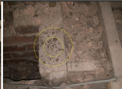
Fig. 6. Bat droppings by loft hatch.
