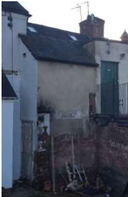
Fig H01: External lime render in poor condition
