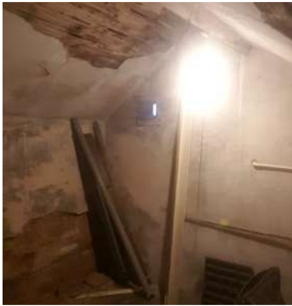
Fig H03: External lath and plaster ceiling in poor condition
