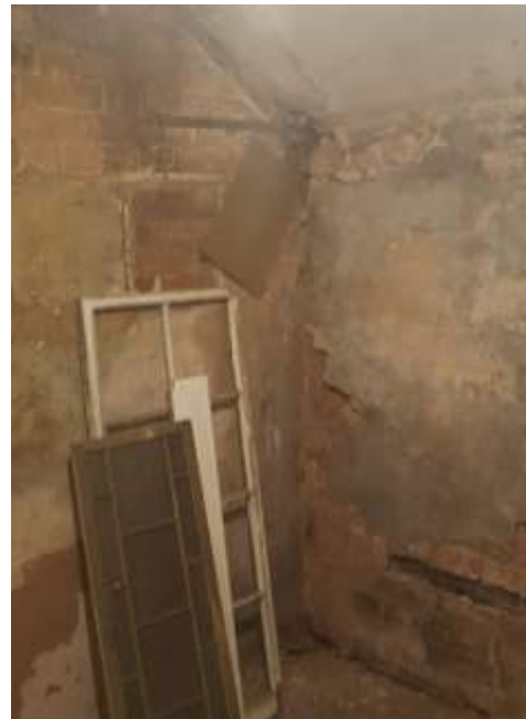
Fig H02: Internal lime plaster in poor condition
