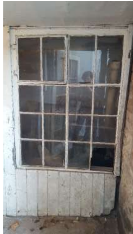
Fig H04: Internal partition wall requiring repairs
