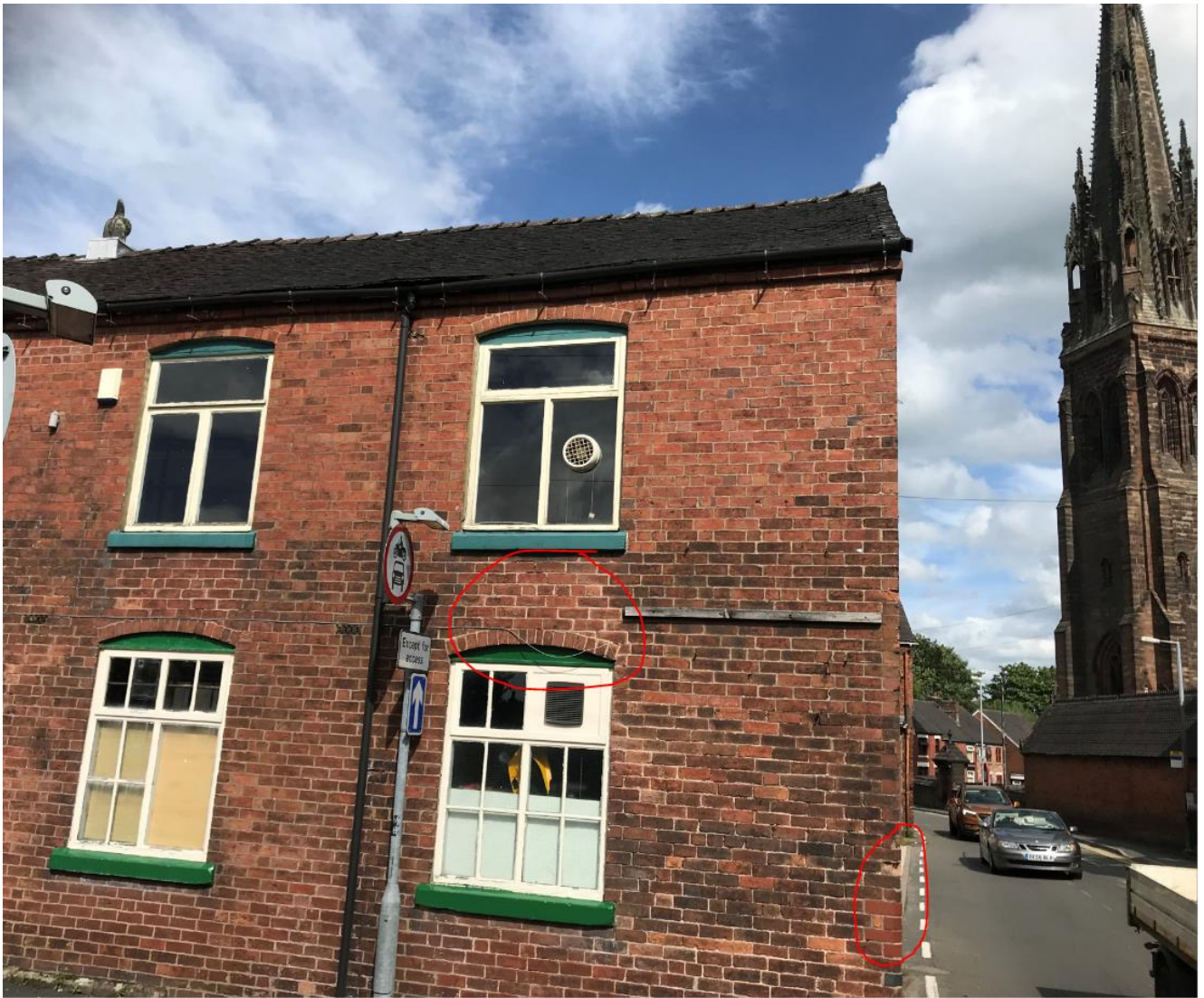
Figure 5 – cracked and repointed brickwork over arch, vehicle-damaged brickwork on corner
