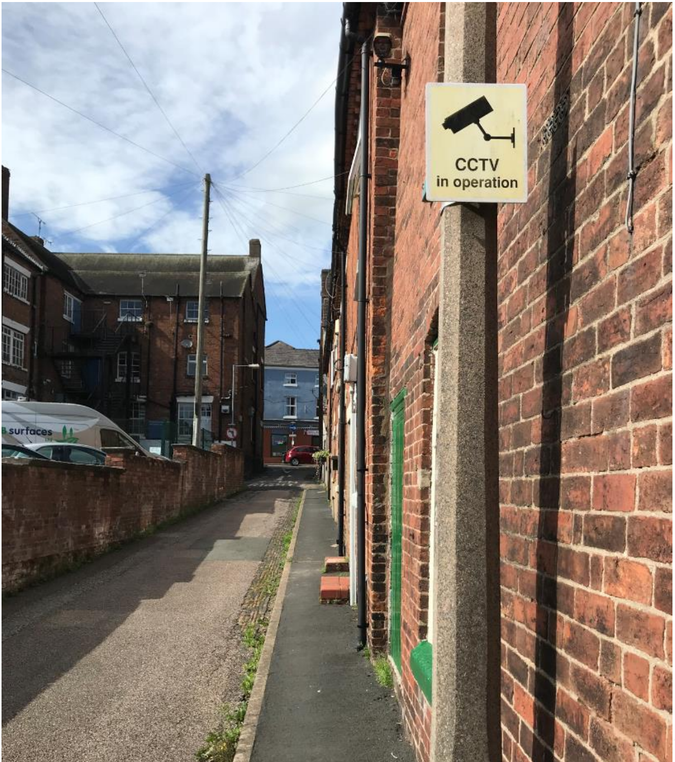
Figure 4 – deviation of front elevation from adjacent plumb building
