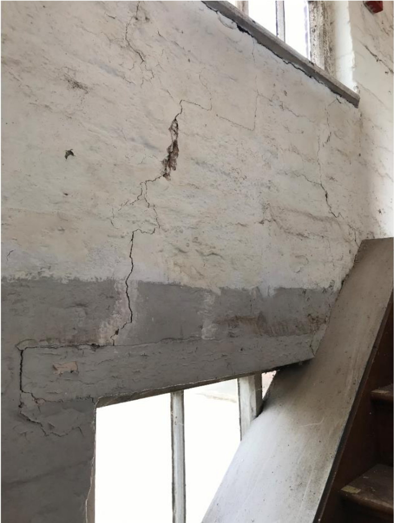
Figure 14 – cracking to rear elevation wall over failed lintel
