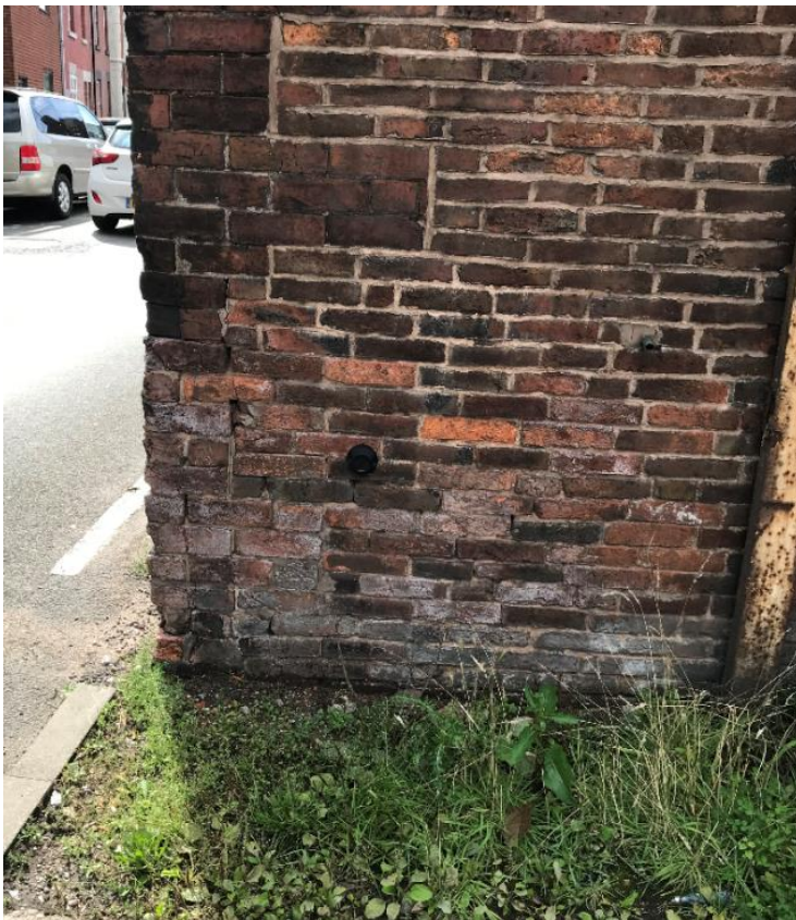
Figure 8 – efflorescence, poor condition of bricks and weed growth at low level
