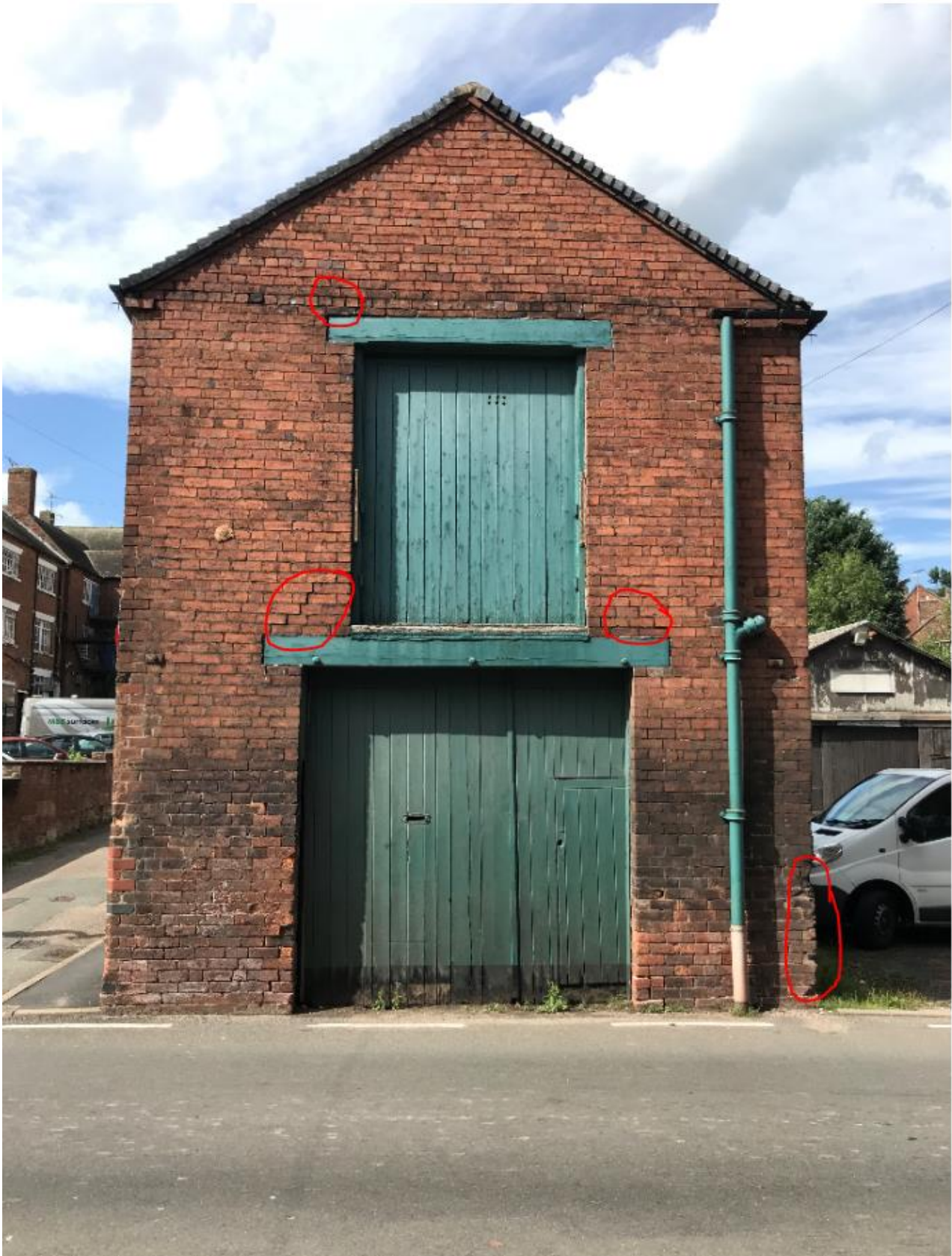
Figure 6 – gable elevation; cracking caused by deflection of lintels, vehicular damage to corner
