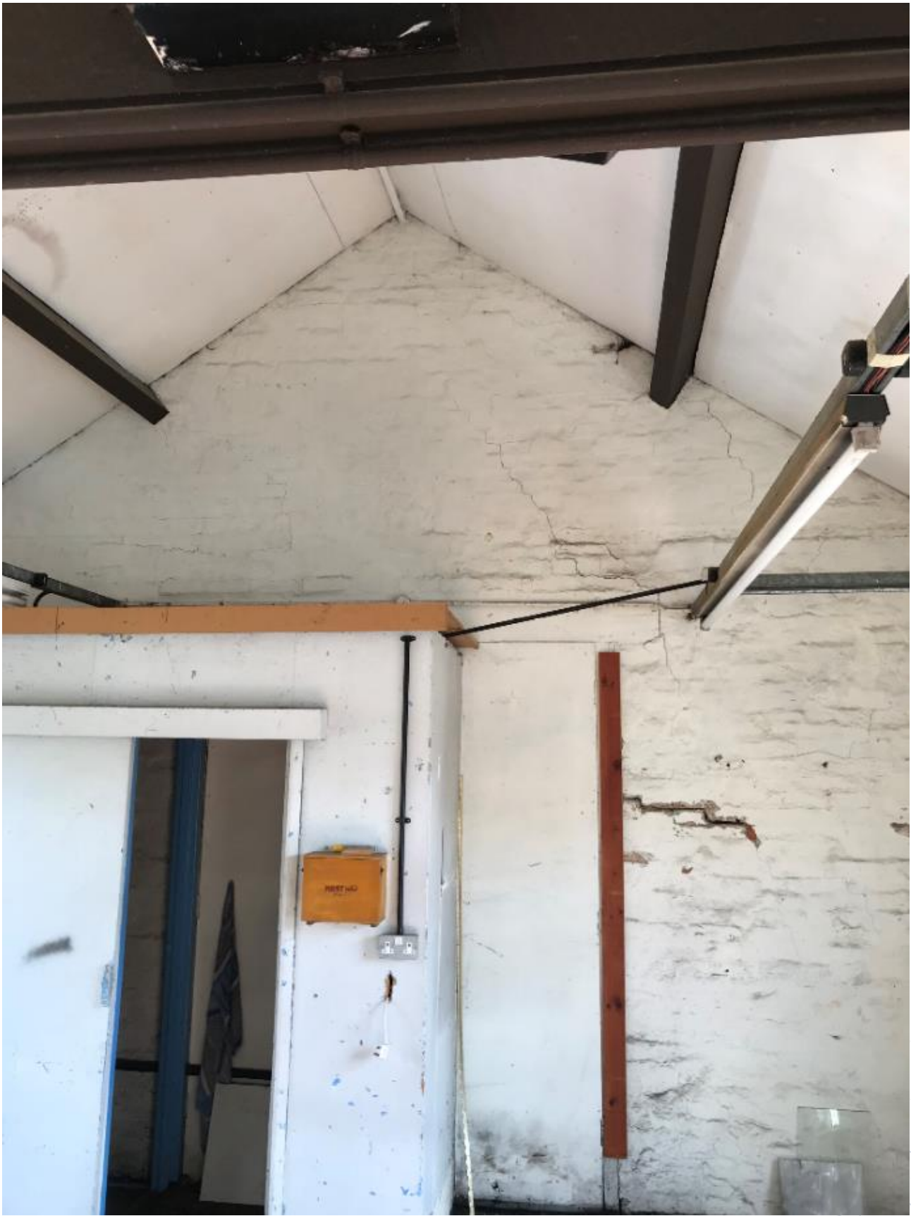
Figure 15 – cracking to gable elevation wall
