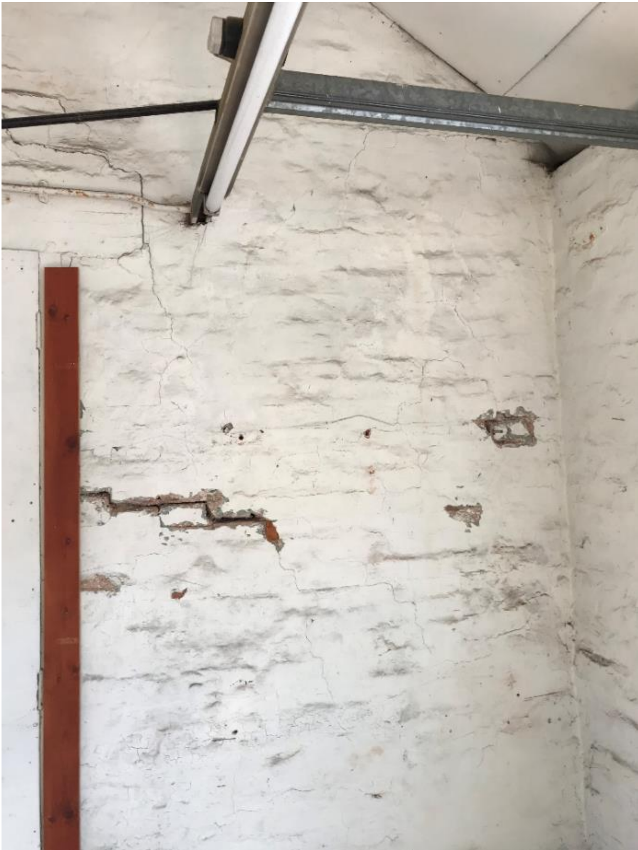
Figure 16 – large and harline cracking in gable masonry
