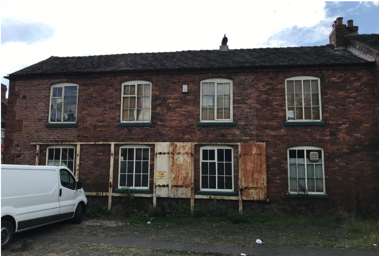
Figure 7 – eastern elevation; unsympathetic toothing and pointing of replaced masonry
