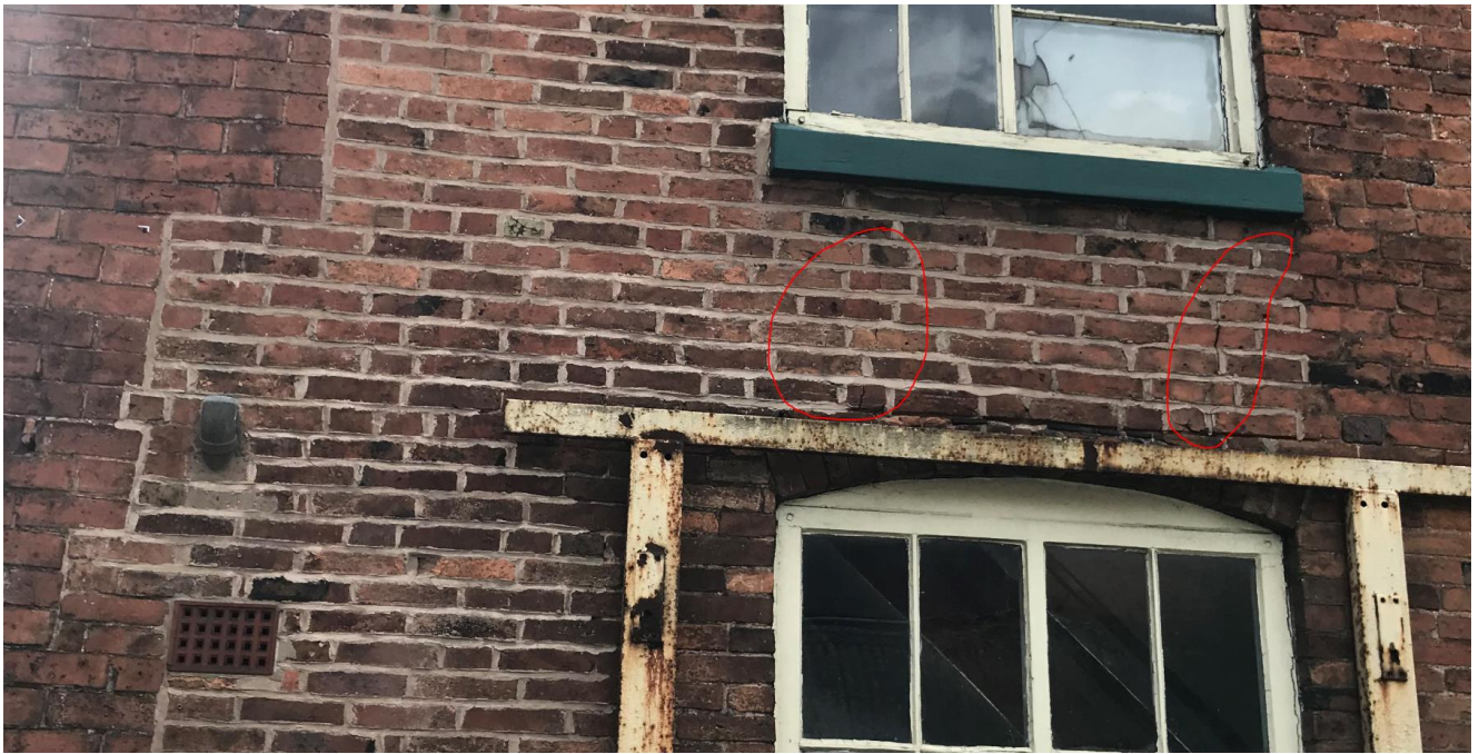
Figure 9 – cracked brickwork over window arch
