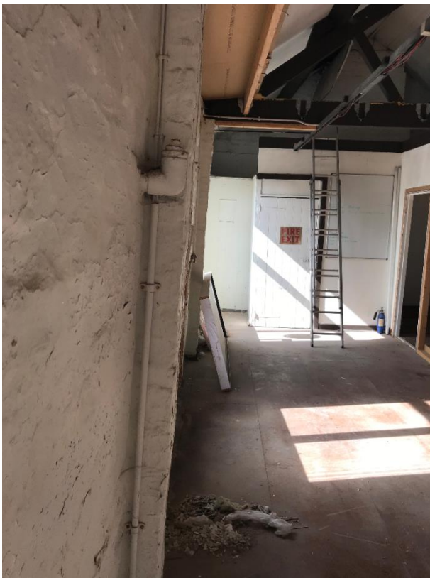
Figure 13 – leaning elevation walls (extent exaggerated)
