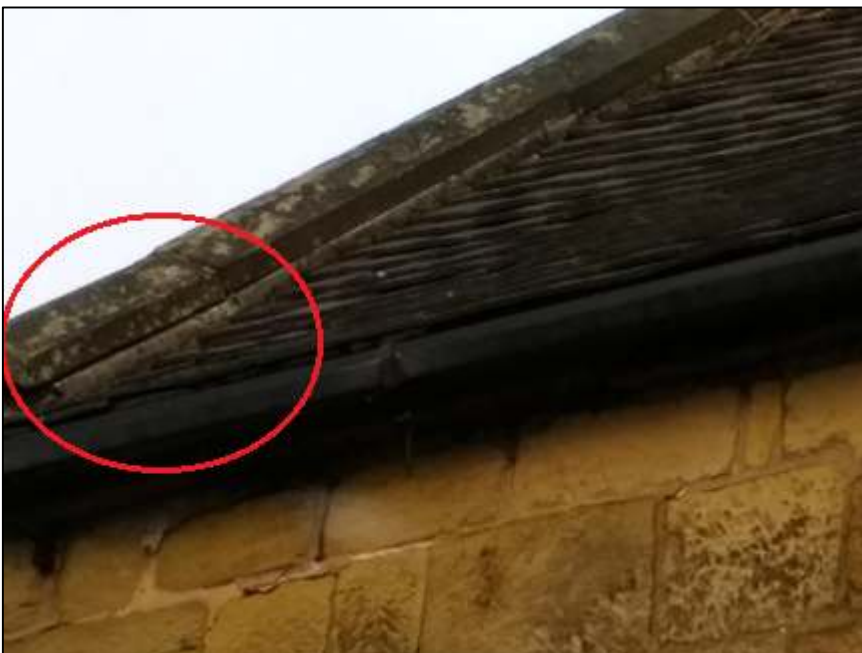
Photographic plate 4: Gap under coping stone on north west elevation
