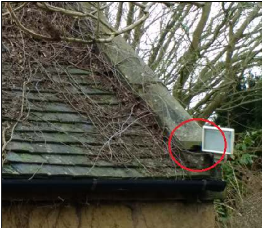
Photographic plate 3: Gap under coping stone on north east elevation
