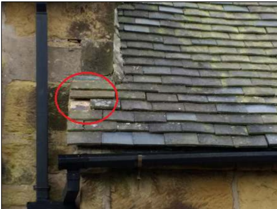
Photographic plate 2: Missing tile on the north east elevation
