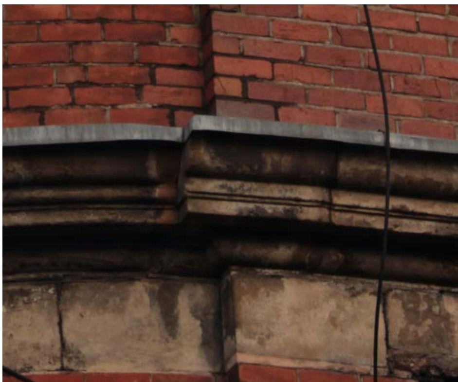
Fig 02 Potential evidence of past movement to cornice. Cementitious mortar repair visible between stones.
