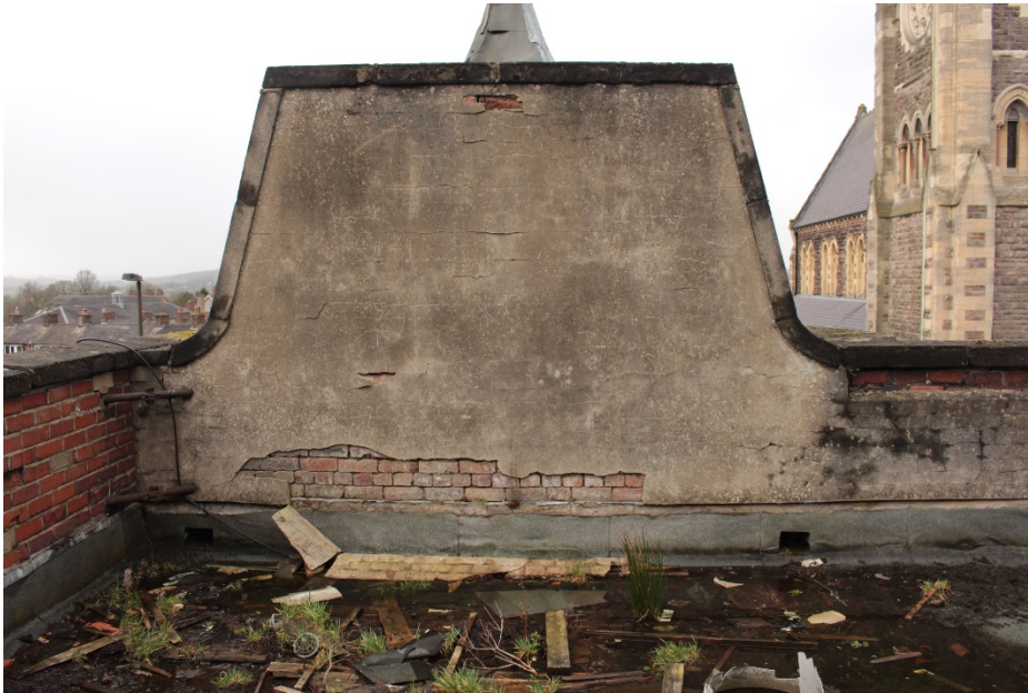
Fig 03 Rear of tall eastern parapet wall, with failing cementitious render. Corner bracing visible to left hand side.
