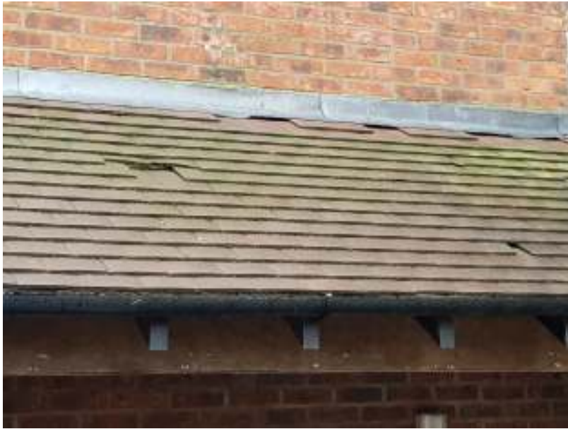
Plate 8; Showing raised, missing tiles and raised flashing potential bat and bird access.
