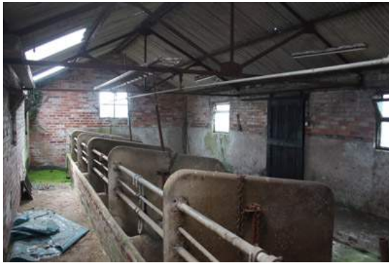
Image 5: Shows internal aspects of Building 2. Note the steel framework and corrugated asbestos roof cover.
