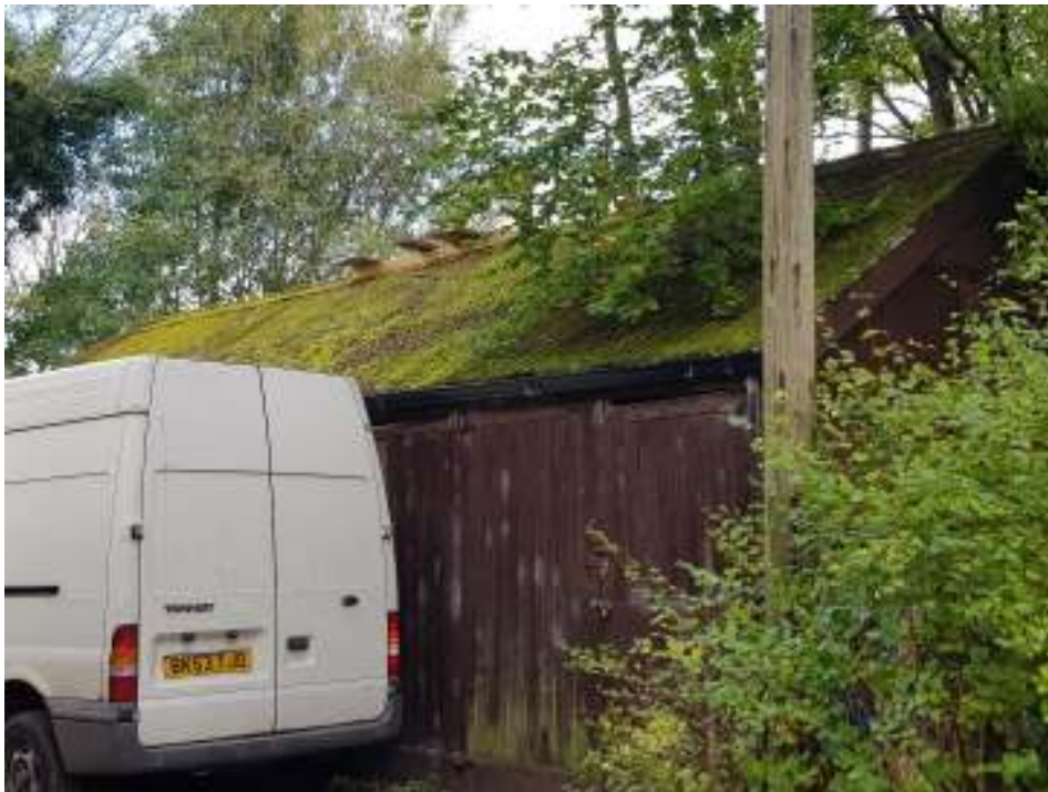
Plate 1: Showing garage, with dominating moss located on the roof.
