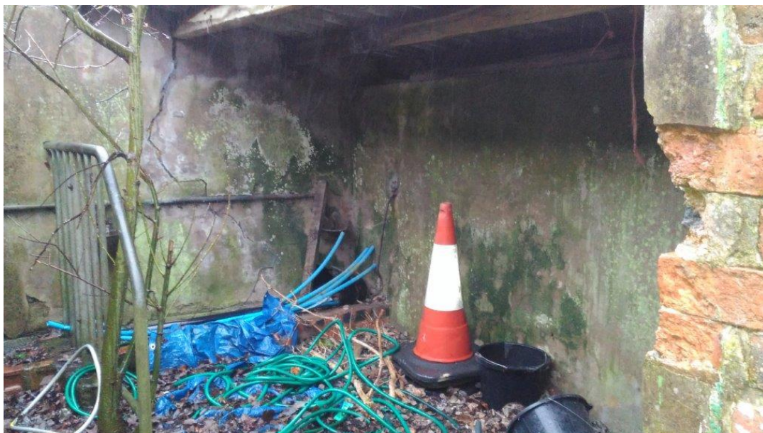
Plate 6: Inside lean-to with broken roof and shallow crack in wall
