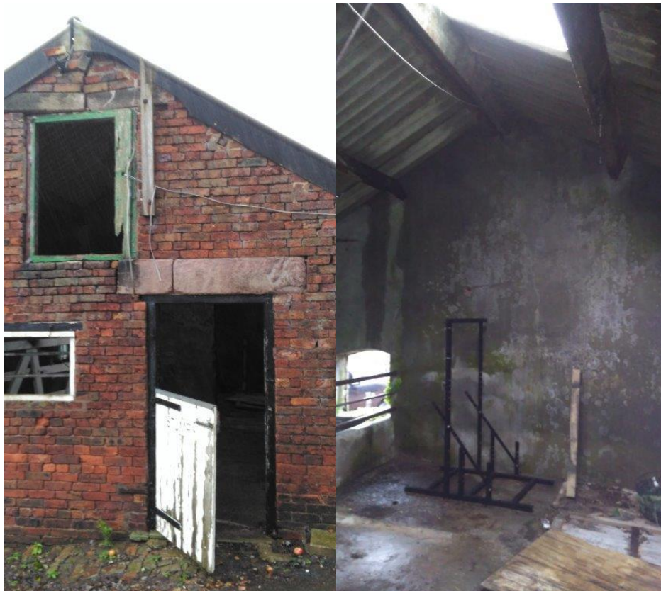
Plate 5: Crevices in brickwork and broken lintel at top of east facing gable wall (left); inside outbuilding (right).
