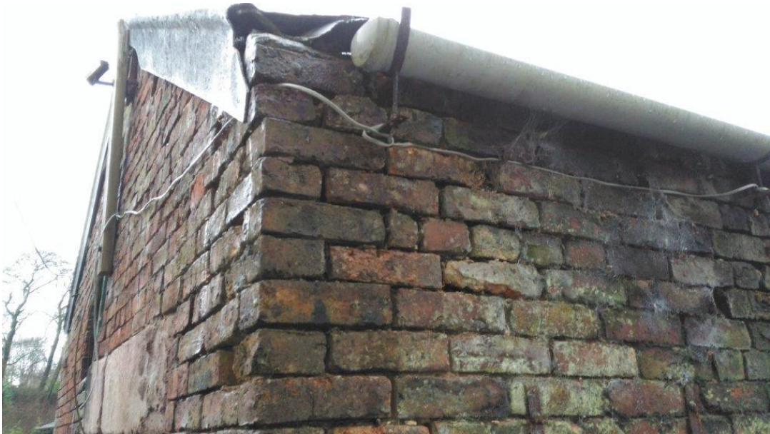
Plate 4: Crevices at top of north wall showing broken roof which is likely to cause water to drain down into the wall
