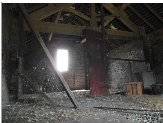
Fig.10. Semi-illuminated SE facing two-storey section roof void showing high infestation of pigeon
