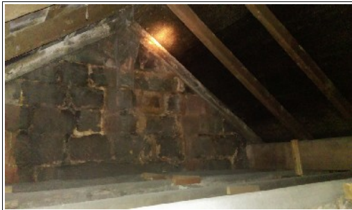
Figure 9. Apex void above dormer section.
