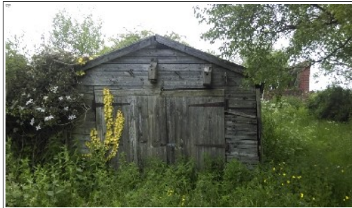
Figure 7. Dilapidated shed on eastern boundary.
