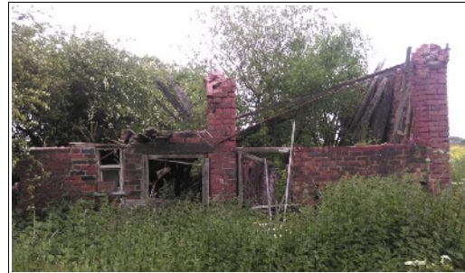
Figure 8. Dilapidated building on NE corner boundary.
