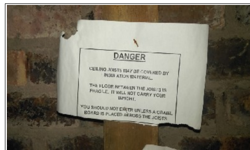
Figure 12. Notice stating fragile roof.
