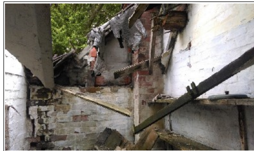
Figure 6. Dilapidated building section on north elevation.
