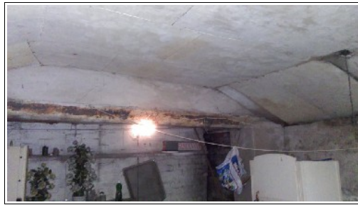
Figure 12. Sealed off apex void above garage section
