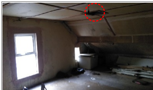
Figure 7. Dormer room in roof section. (NB. Access loft into apex void- red dash).
