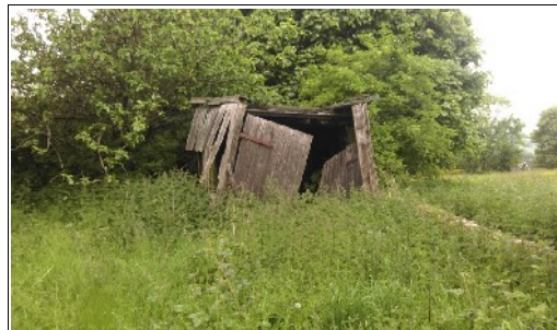
Figure 9. Dilapidated shed on northern boundary.
