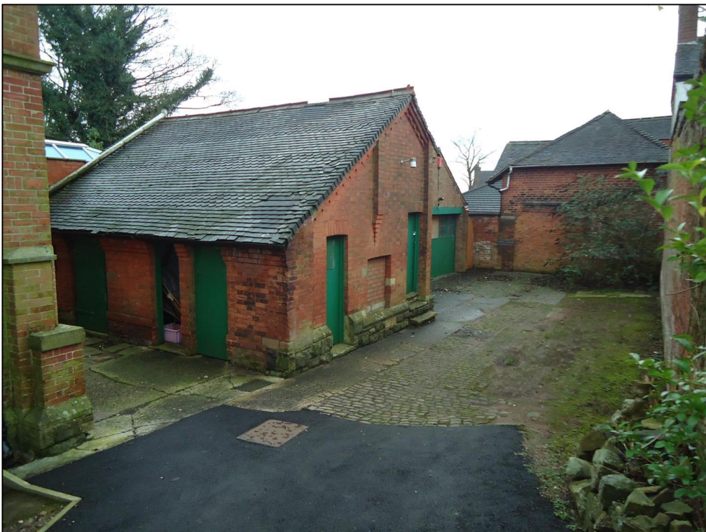
Photograph 2 . Existing dilapidated stores/garage
